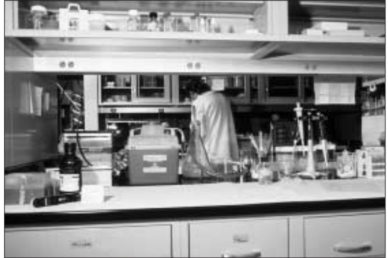
Standard devices installed in aluminum raceway mounted under reagent shelf in medical center lab.
