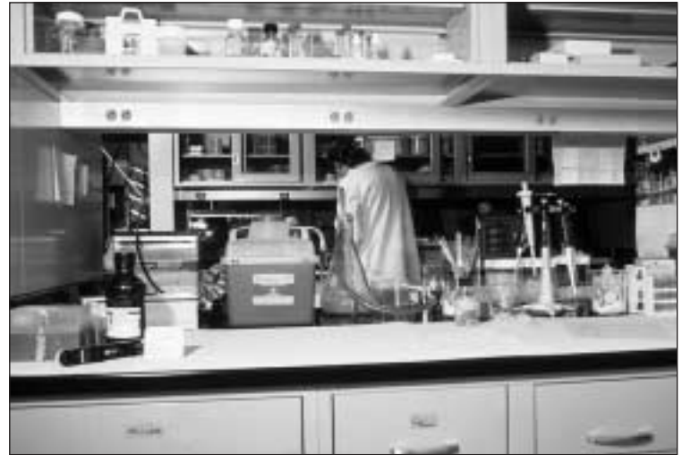
Standard devices installed in aluminum raceway mounted under reagent shelf in medical center lab.
