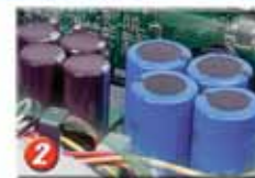
74,600µf of Capacitance Creates Enormous Amounts of Reserve Energy
