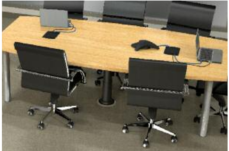
A conference room with Under Table Cable Management and Meeting Room Transition Channel installed to manage cabling below the work surface.
