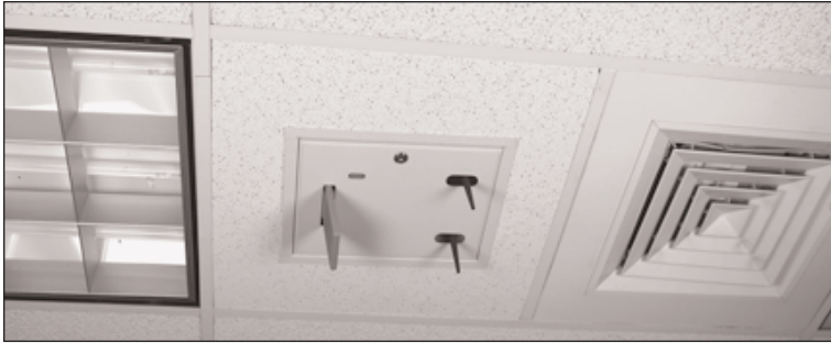
Application in air handling space.
