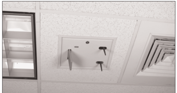
WAPE Wireless Access Point Enclosure installed in a drop ceiling.
